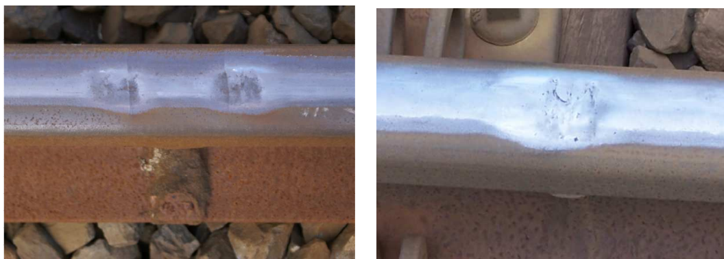
(a) A squat at a thermite weld
