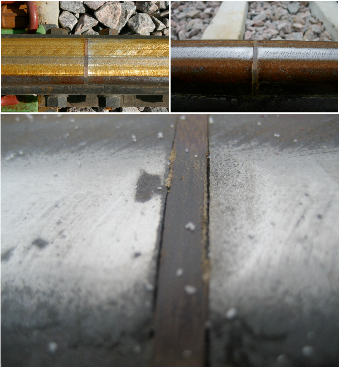
Figure 5 Damage evolution of an insulated joint. From top to bottom: 2008-06-11 (the week before the start of operational traffic, but after grinding), 2008-08-20 and 2009-02-20.
