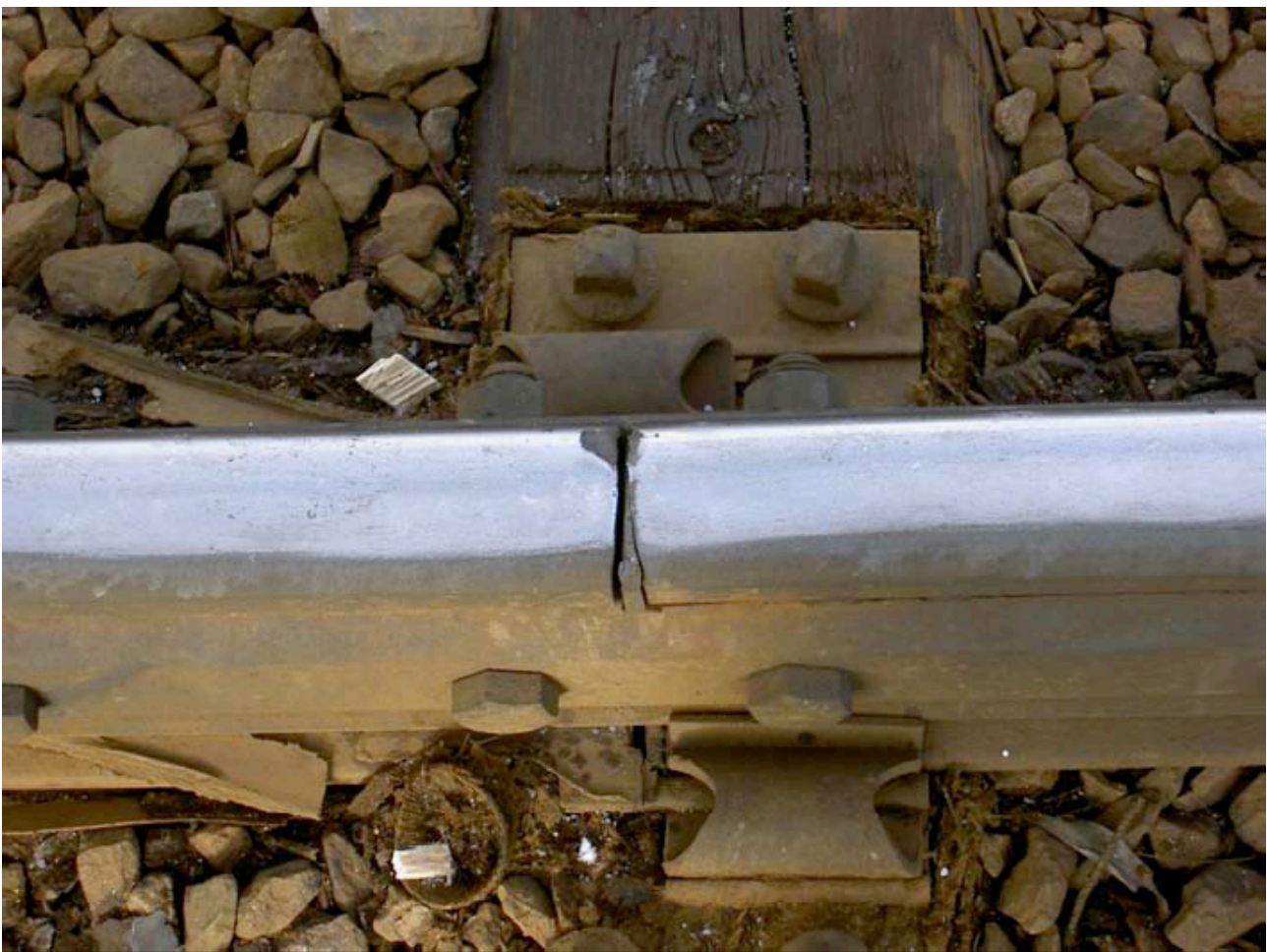
Figure 2 A severely deteriorated insulated joint.
