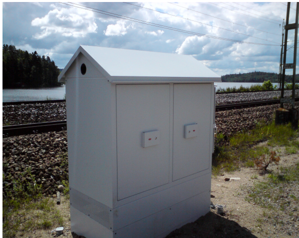
Figure 5.1: Cabinet in place. The round hole up to the left is for the camera based train identifier.
