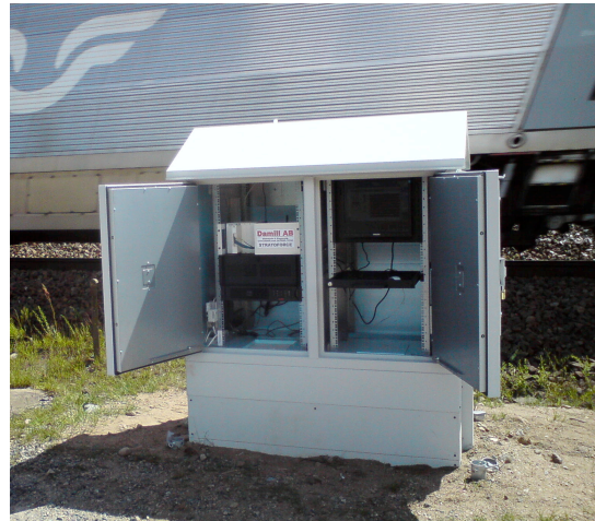
Figure 5.2 Cabinet with open doors. Computer and sensor electronics are placed to the left while the consol is placed to the right.
