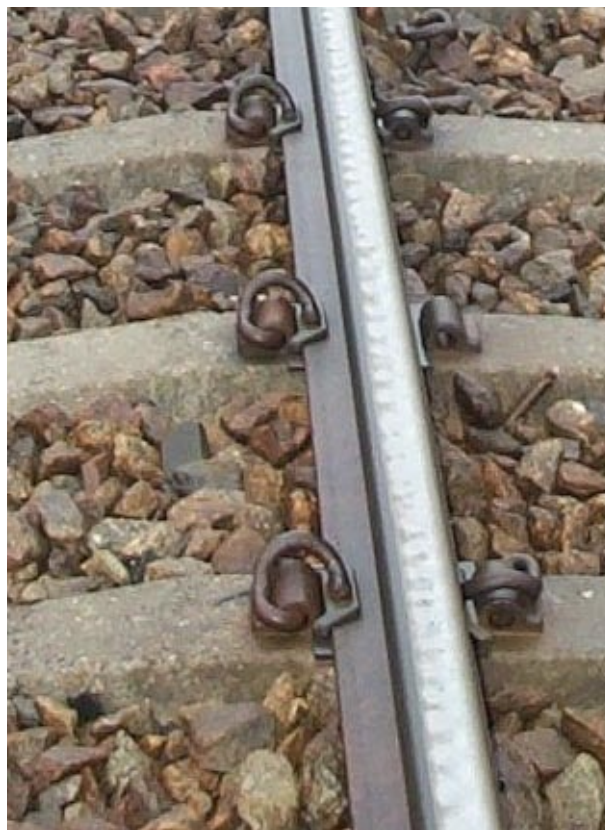
Short pitch corrugation at Kilsmo on the Western Main Line in Sweden
