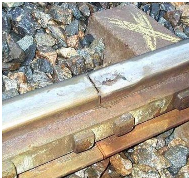
Damaged insulating joint at Järna south of Stockholm. Running direction of train is from right to left. Measurements in project SP11 showed that the wheel of an X2 train travelling at 185 km/h flies over the cavity and then bounces twice with a peak contact force of 350 kN
