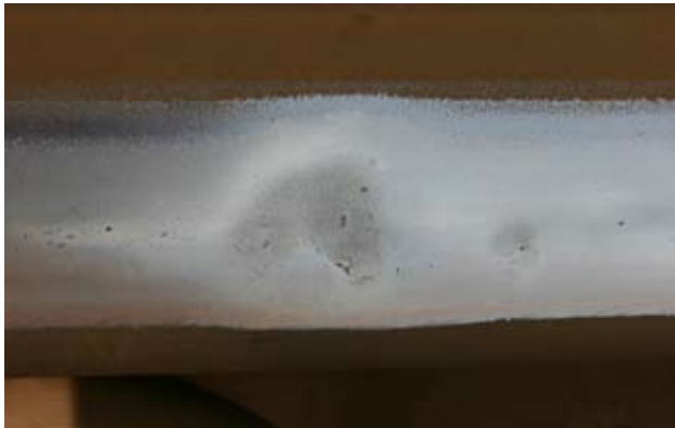
Typical squat-like defect found on a metro line rail in Stockholm (Sweden). Two distinct lobes are visible. Also note the V-shaped surface breaking crack and the slight widening of the running band. Photo by Robin Andersson
