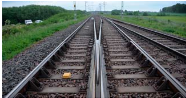
Crossing panel with accelerometer (yellow box). Image from the Southern Main Line in Sweden
